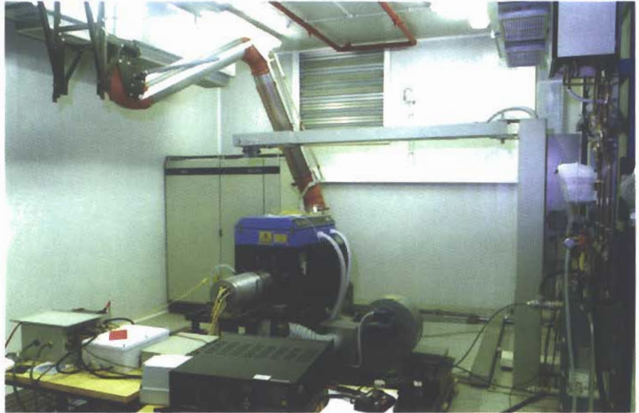
120 kW motor test room
