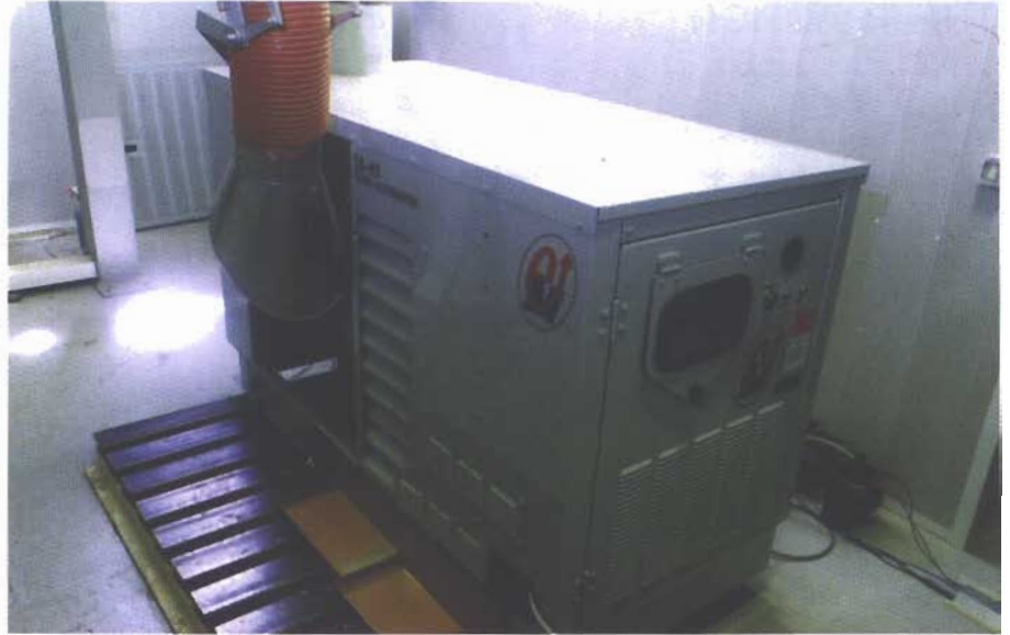
Generator test room (fuel cells, motor generators, etc.)
