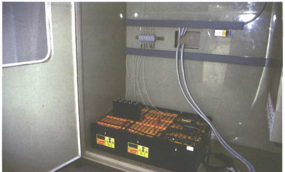
Battery test room
